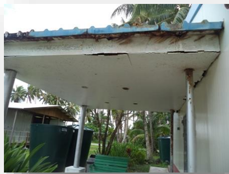
Figure 1: need of repair at the entrance to the cafeteria.
